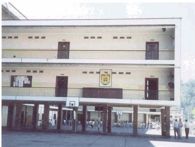
This school in Quito has a “soft” first storey that lacks infill walls, an example of a common structural deficiency.
