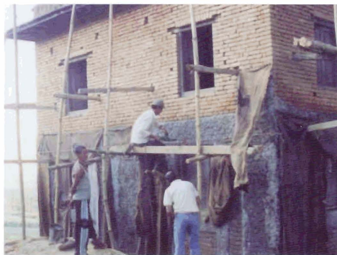
Kathmandu Valley: GHI’s Nepali partner, the National Society of Earthquake Technology (NSET) trained masons to retrofit the school of Nankhel village.
