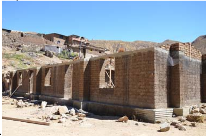
Geomesh is applied to both the interior and exterior walls. Courtesy of GHI/Stanford/PUCP
