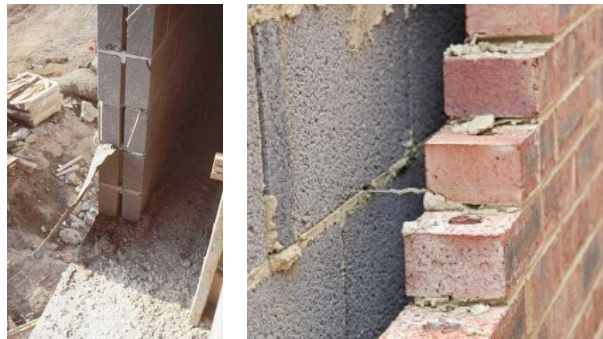
Figure 19. A cavity wall (photo on the left from Syracuse University libraries, photo on the right from anewhouse.com.au )
