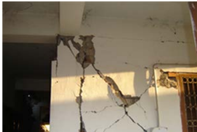
Figure 8. Column shear damage caused by interaction between frame and infill during the 1988 Udaypur, Nepal earthquake. (Photo credit: World Housing Encyclopedia, Report 145)
