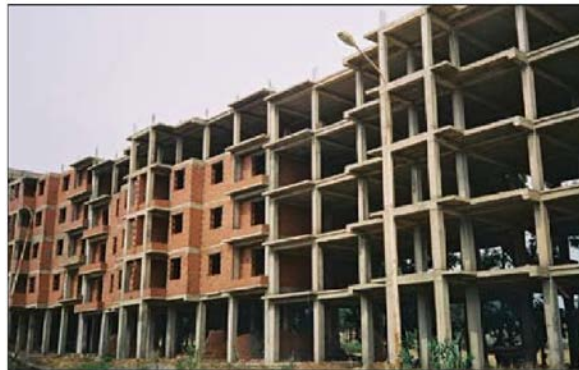
Figure 11. Residential buildings with hollow clay tile masonry infill under construction in Algeria (Photo credit: S. Brzev, World Housing Encyclopedia, 2013).
