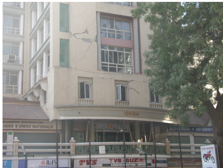
Figure 21. Diagonal shear cracks in the wall indicate that it provided resistance and energy dissipation during the 2001 Gujarat, India earthquake. (Photo and description by Rakesh K. Goel, California Polytechnic State University)
