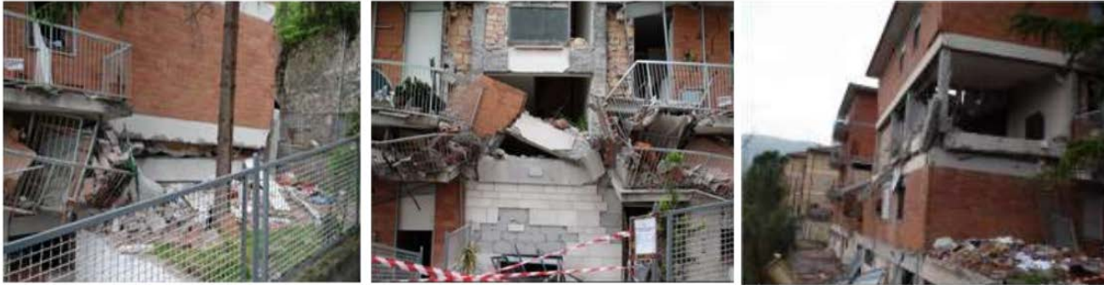
Figure 4. Story collapse due to infill failure, 2009 L'Aquila, Italy earthquake (Photo credits: K. Mosalam)
