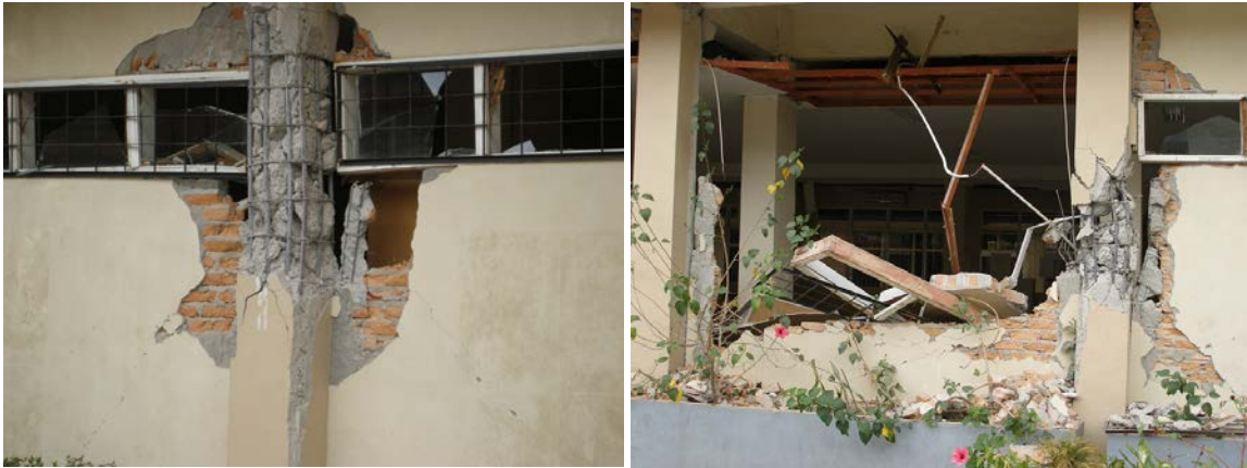
Figure 6: Schools with shear damage caused by the short-column effect following the 2009 Padang, Indonesia earthquake (Photo credits: Tim Hart, Lawrence Berkeley National Laboratory)
