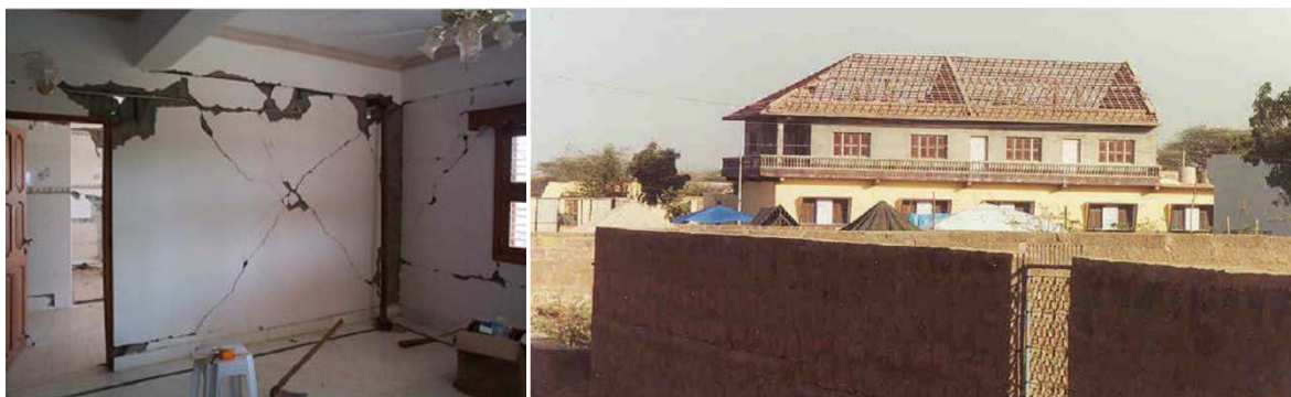
Figure 23. Infill panels prevented collapse of the whole structure during the 2001 Gujarat, India earthquake. (Source: Patel et al., 2001)
