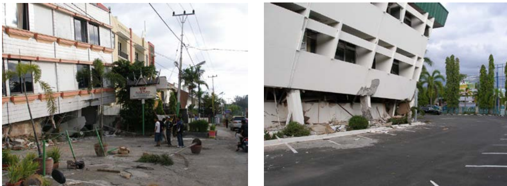
Figure 3. Soft-story collapse of infill buildings from the 2009 Padang, Indonesia earthquake (Photo credits: Tim Hart, Lawrence Berkeley National Laboratory)
