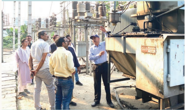
India: GHI-led team shares recommendations to improve the seismic resilience of power infrastructure. Preventing long & widespread outages during disasters can save lives.
